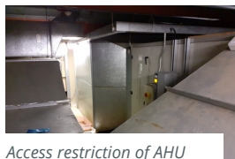
Access restriction of AHU
