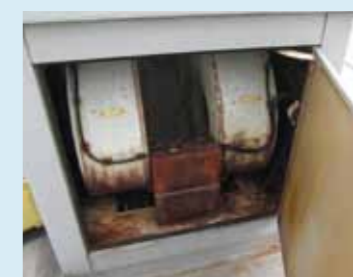
Failed and tired units
