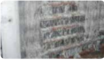
Severely corroded coil
