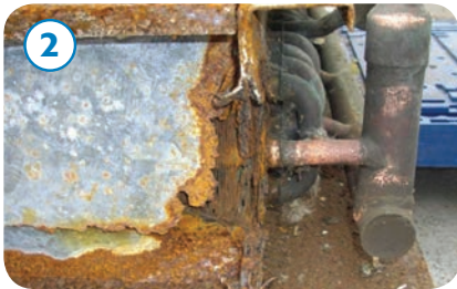
Condition of condenser coil when removed.
