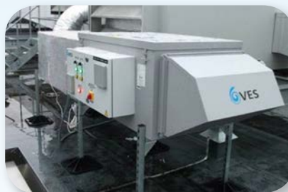
VES Temporary Heating AHU on Site
