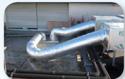
Temporary Ducted Heating System
