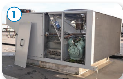
1 AHU Before with failed compressor
