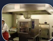
▶ Restaurant Kitchen Ventilation
