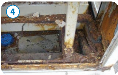
True condition of casework with condensor coil removed
