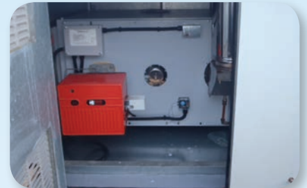
New gas heater
