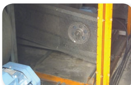
Unit with old belt driven fan
