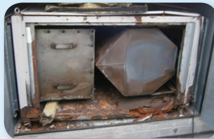
Old gas heater
