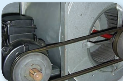
Unit with old forward curved belt driven fans
