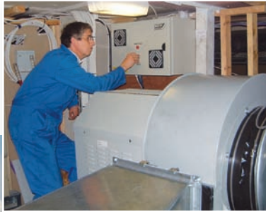
Workhorse fan with inverter control
