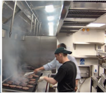
Kitchen hood with Grease Grabbers
