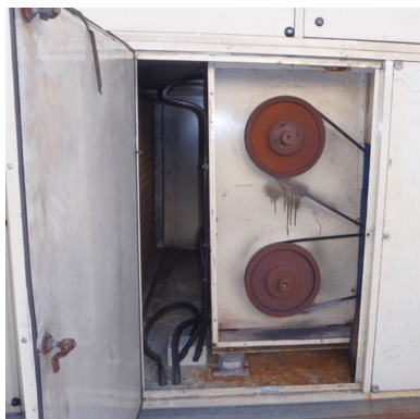
Before - inefficient belt driven fans
