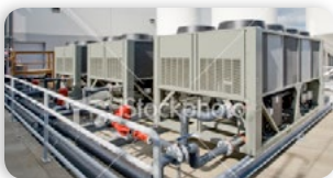
Heat Transfer - Cooling and Refrigeration
